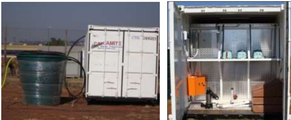
Fig 19: Containerised waste water treatment plant
